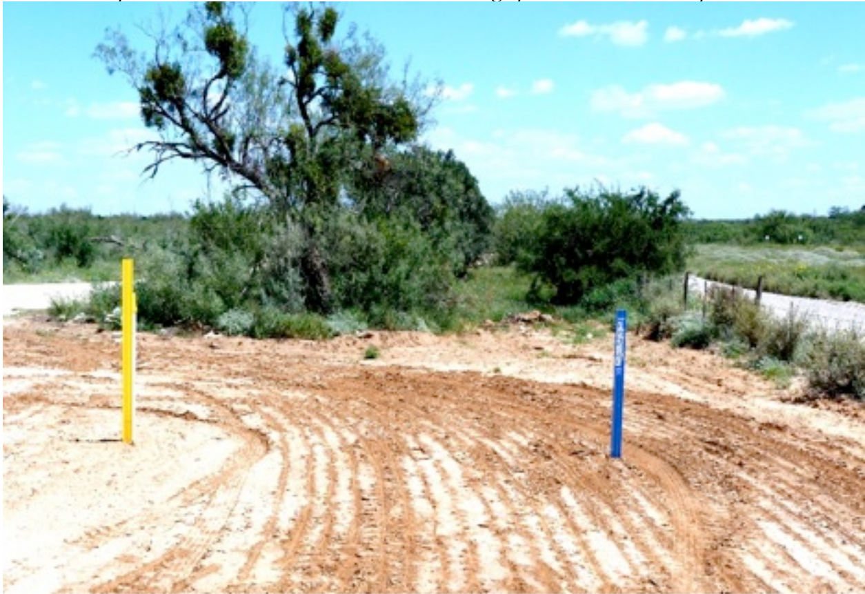
Figure 1. Small riparian area that was bored to save the large persimmon and mesquite trees.
